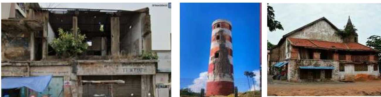
Figure 2-11 Image of old buildings, town hall & light house in damaged condition
